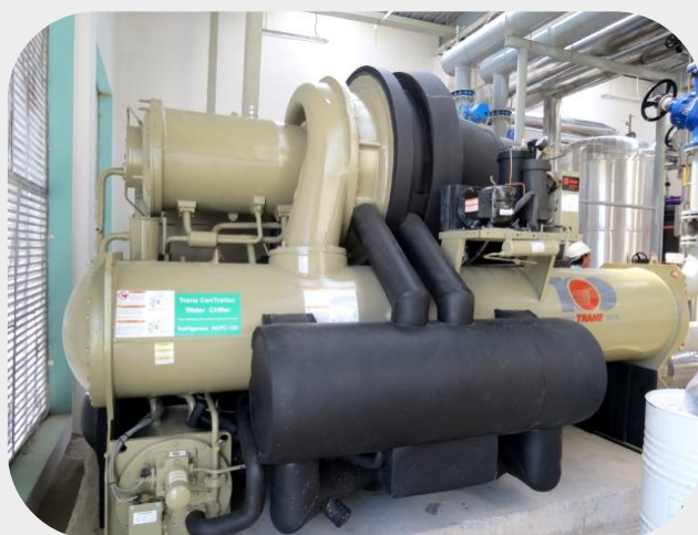
Chiller li tâm /Centrifugal Chiller
