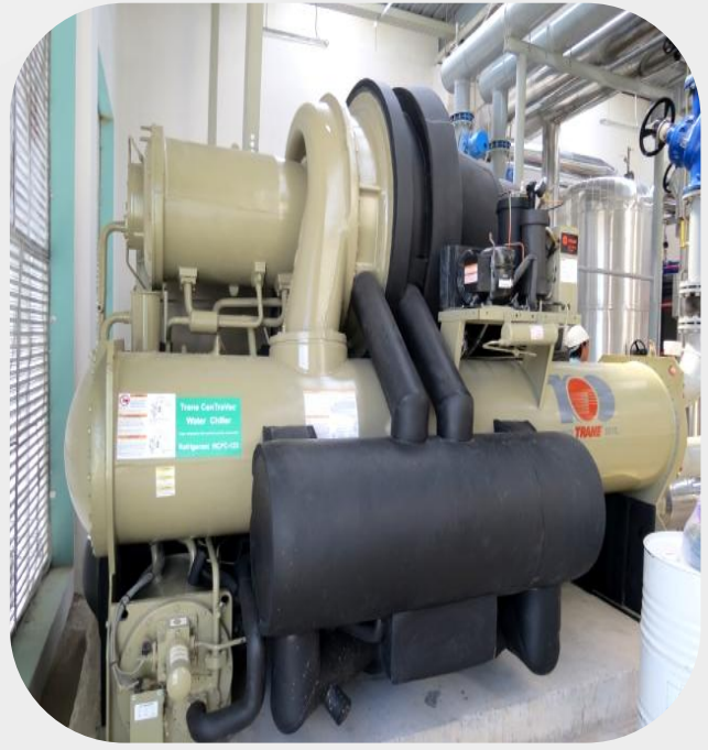
Chiller li tâm /Centrifugal Chiller
